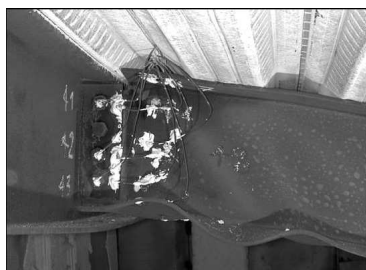
Fig. 5 - Local buckling after 2003 Cardington experimental fire 5 .
