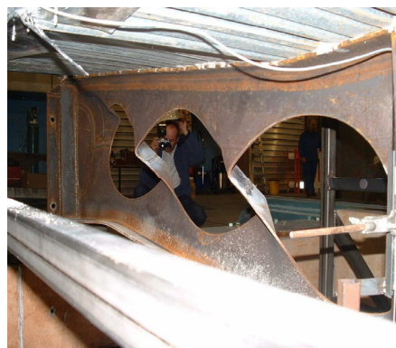
Fig.2 - Beam failure at the post web
