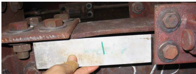
Figure 12. Buckling of beam bottom flange of C1-2 after test
