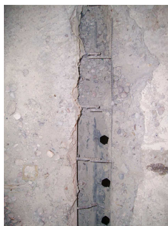
b- State of the reinforcement joint at the location of the crack after cooling
