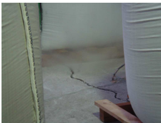
a- State of the cracking at central part of the floor
